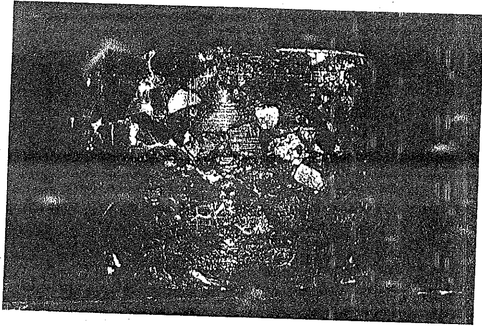
Plat 11 Close view of core confirming full depth cracking in Asphaltic layers.
